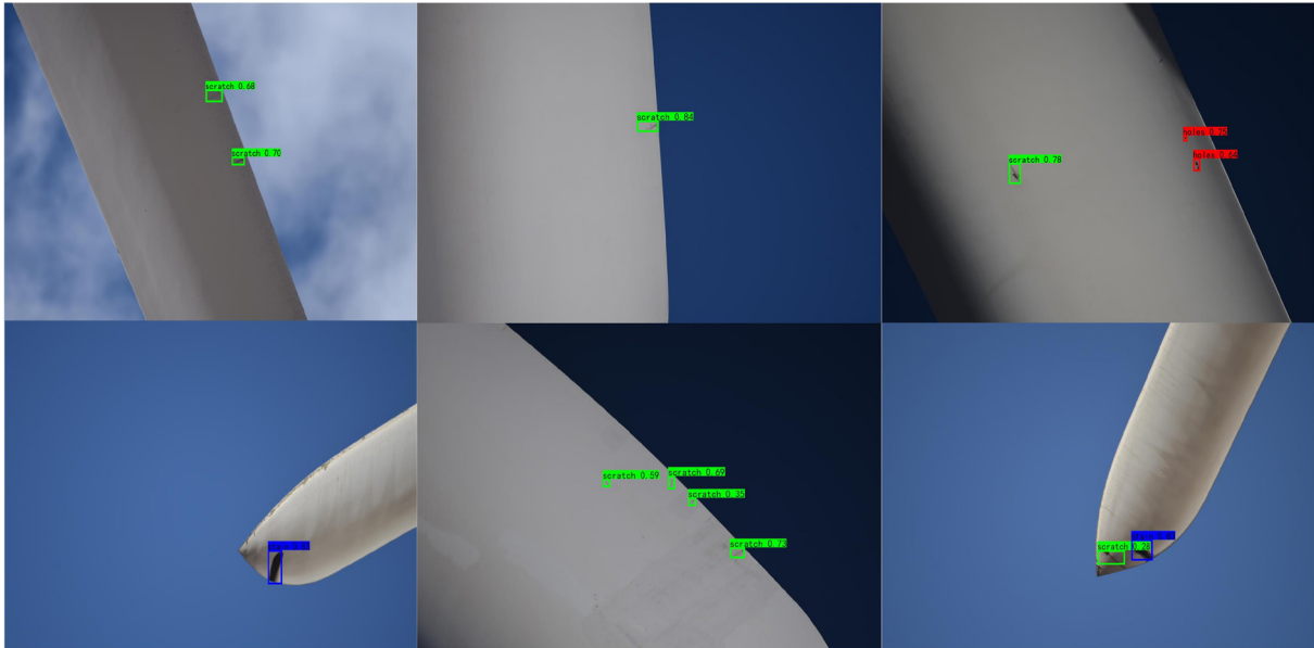
Fig. 9. Image of surface defects of wind turbine blades identified
